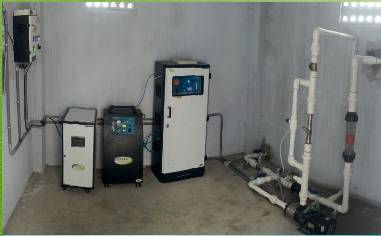
25 m 3 /h Online System Installation
