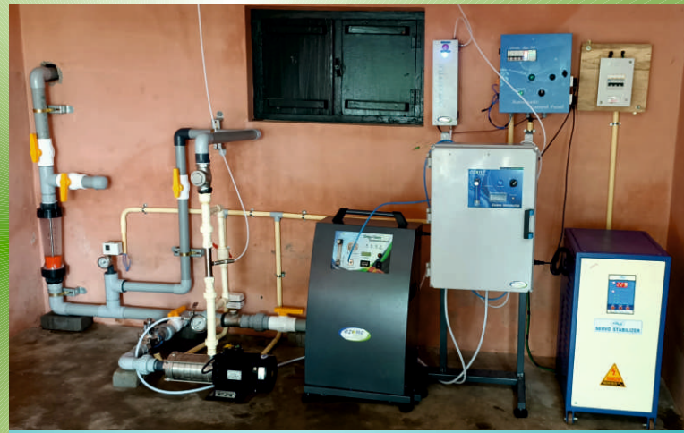
15 m 3 /h Online System Installation
